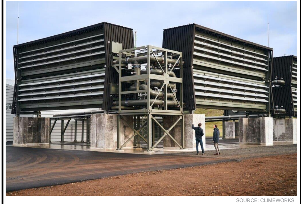
Figure 88: The Climeworks Orca DACCS plant in Iceland (capacity 4 ktpa of CO 2 )
